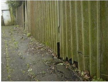
Figure 1: Asbestos fence panels
