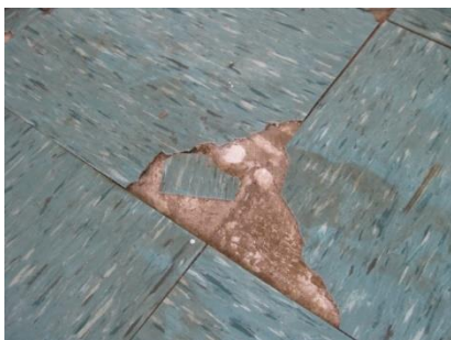
Figure 7: Asbestos vinyl flooring
